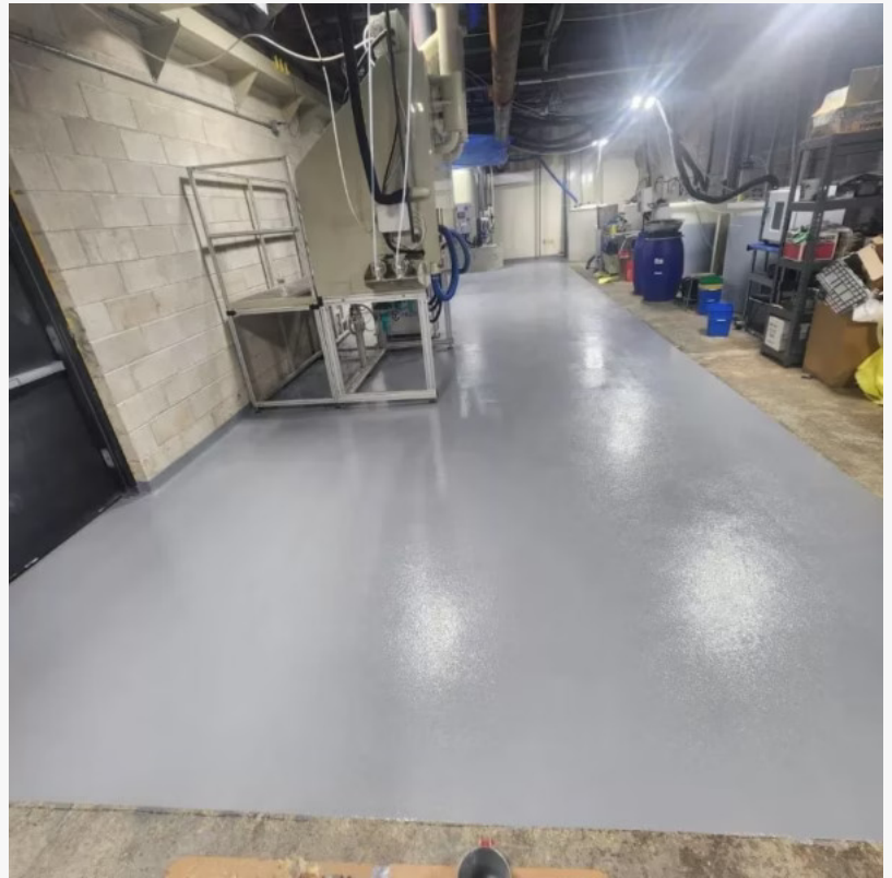
Mechanical Room Flooring
