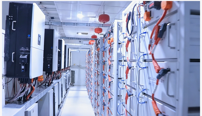
2.49MWh Industrial BESS Project Successfully Commissioned in Yemen with GSL Energy High Voltage Battery Technology
