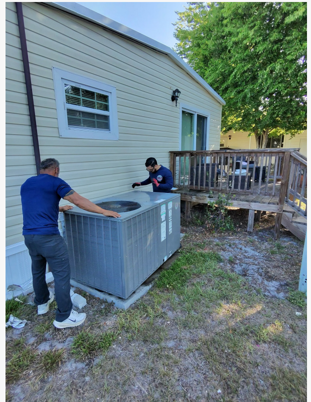
M&R Air Conditioning team
