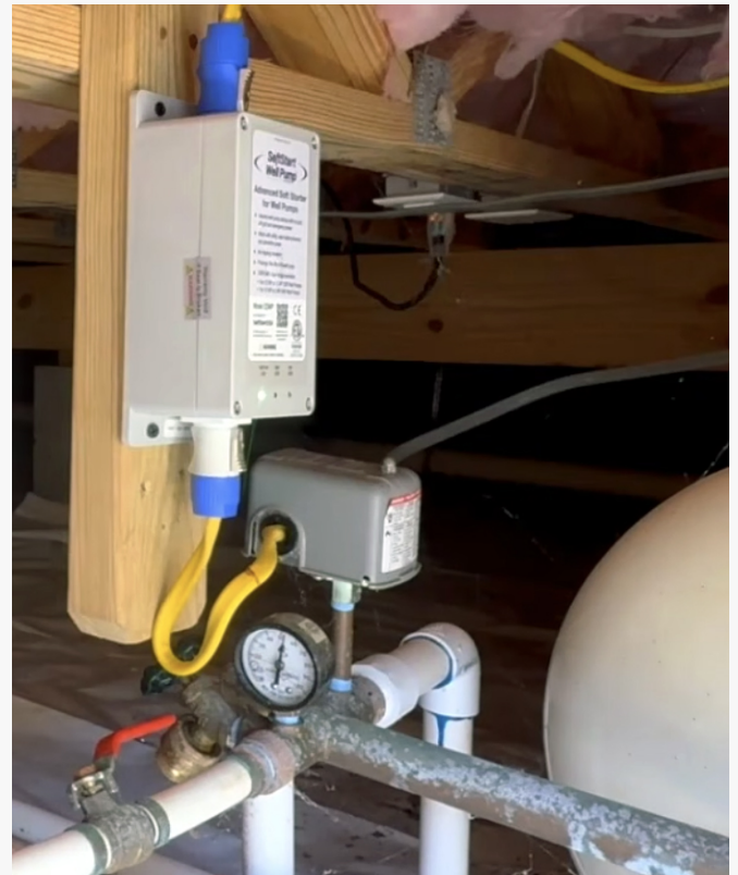
Well pump soft starter installed next to pressure tank
