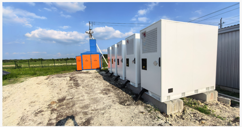
Field-proven 800V BESS deployments across European solar-plus-storage portfolios, with over 300 Galaxy 418L units in commercial operation.
