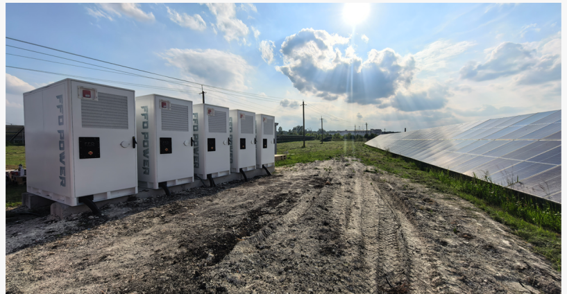
Galaxy 418L 800V battery energy storage units deployed at an 800V solar farm, enabling direct low-voltage integration without a dedicated matching transformer.
