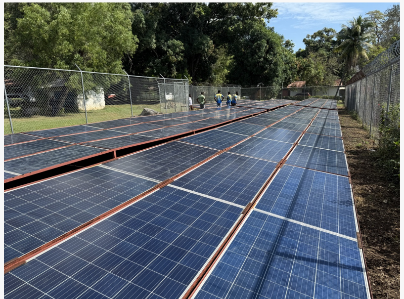
Solar panels at Bethesda Medical Center in Haiti are part of a system that provides lights overnight in the emergency department. Additions to the system are urgently needed now to reduce the amount of fuel still required for the diesel generator during peak hours
