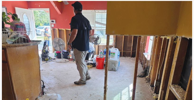
ADRN Executive Director Dr. Dwight Bailey surveys a flood-damaged home in Chula Vista as teams prepare for debris removal and recovery work.
