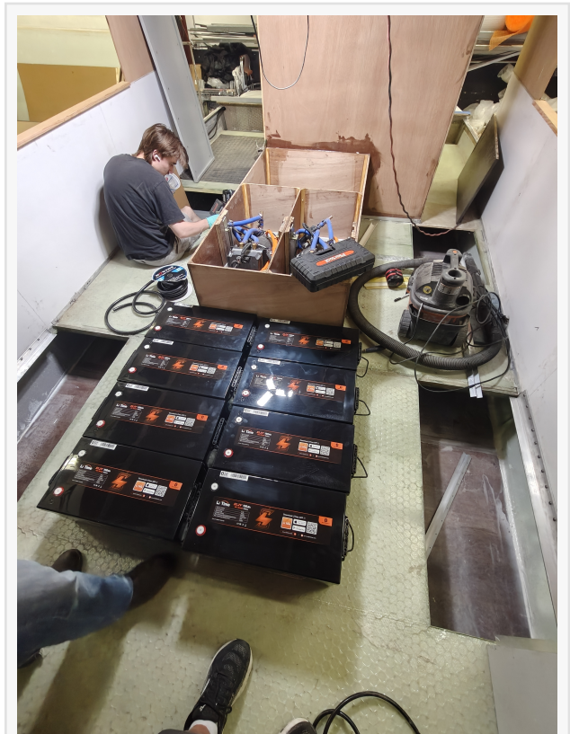
LiTime 12V 100Ah lithium batteries staged during the electric powertrain installation aboard Wada Hoppah's Just Get On, part of the battery bank that powers the ferry.
