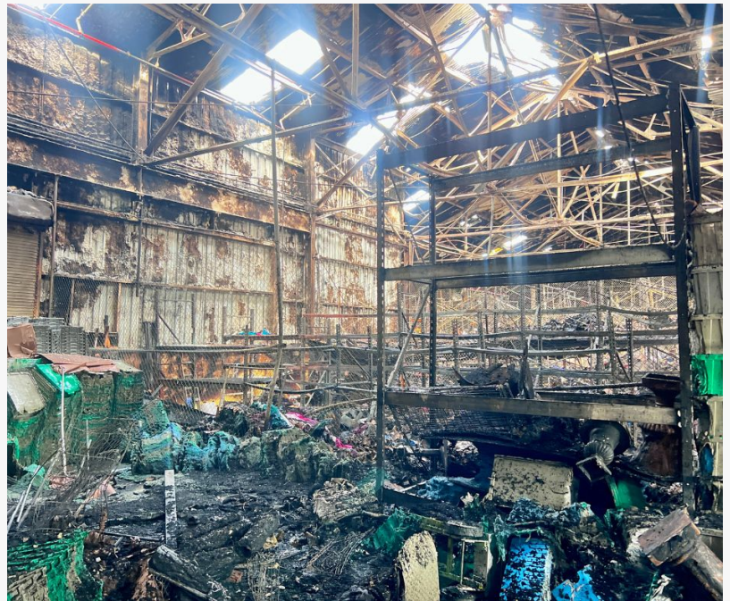
Inside the Cool Hand Movers warehouse after January 21 fire.
