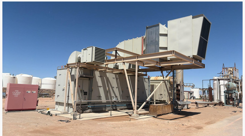
6.5 MW Solar Model 70 natural gas-fired turbine generator
