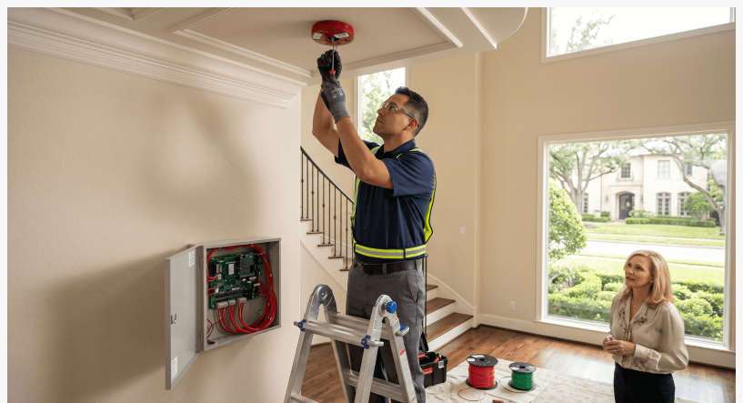
Fire Alarm System Services in River Oaks Houston
