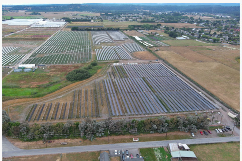
Picture of the largest new build solar and storage project on California's North Coast.
