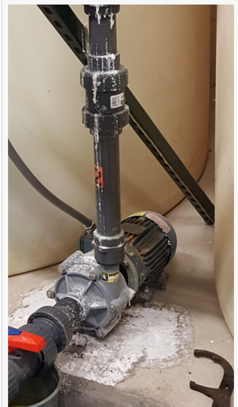
Chlorine leaks in water treatment fitting before applying LOX-8 thread sealant.
