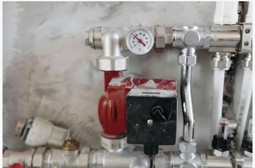
HVAC and plumbing services
