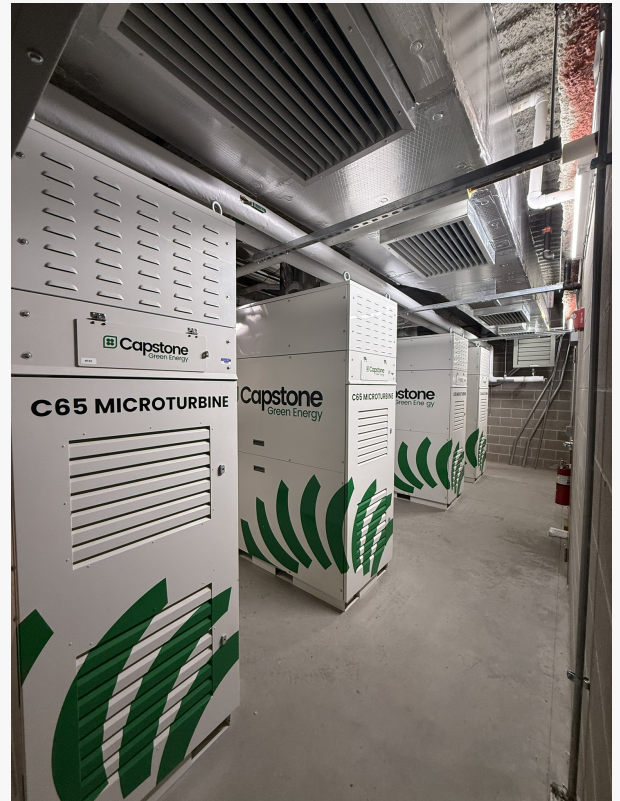
The hospital's high-efficiency energy system generates both electricity and heating on site.
