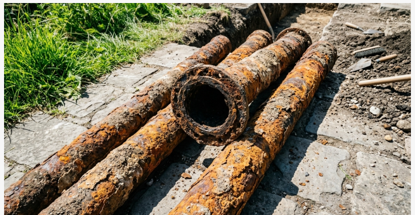
Decades underground take their toll: corroded, narrowing cast iron sewer pipe.
