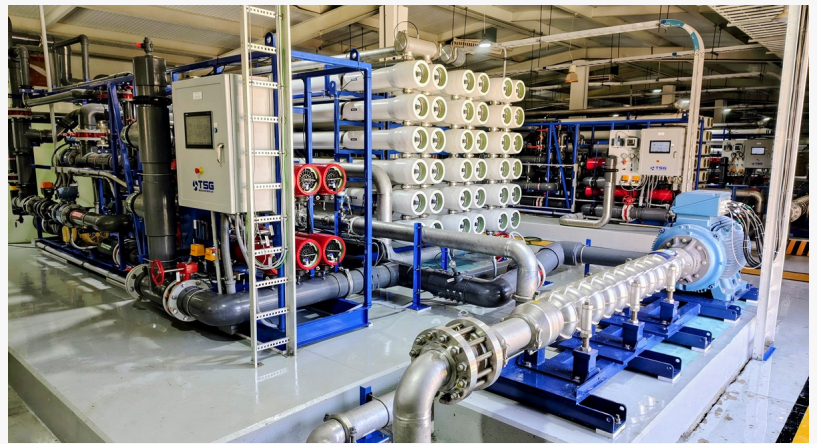
TSG's newest high recovery addition to a facility in Baja California Sur
