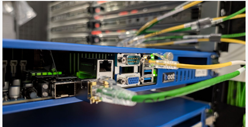
ReliableSite server and network infrastructure. The company has expanded its dedicated server platform to Amsterdam and Querétaro, Mexico.
