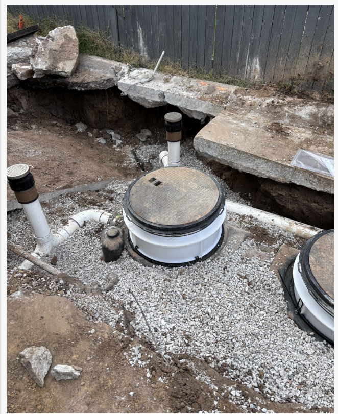
A Tulsa restaurants grease trap
