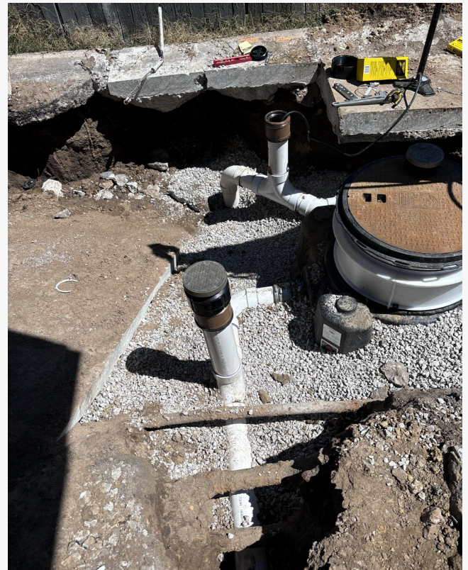
A Tulsa restaurants grease trap
