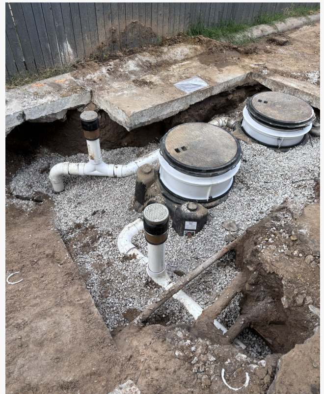
A Tulsa restaurants grease trap
