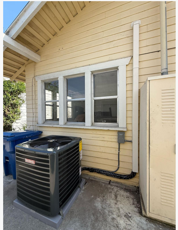
Outdoor air-conditioning condenser beside a home. Equipment photograph for illustration.
