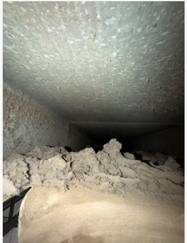
Dust and debris inside an air duct. Original job photograph supplied by Monarch Air Duct Cleaning.
