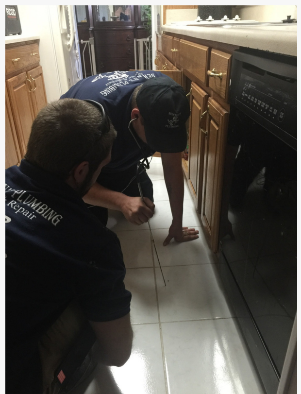
Newman's Plumbing technicians perform a camera inspection to diagnose a plumbing issue.
