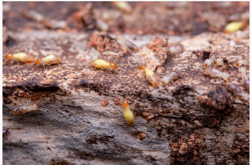
A working colony of subterranean termites moving across the eroded surface of a timber, with workers and soldiers visible among the damaged grain.
