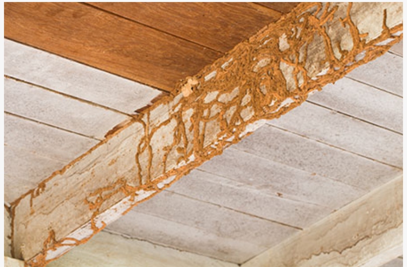
Termite mud tubing running the length of a ceiling joist, built up in branching trails across the painted timber and the boards above it.
