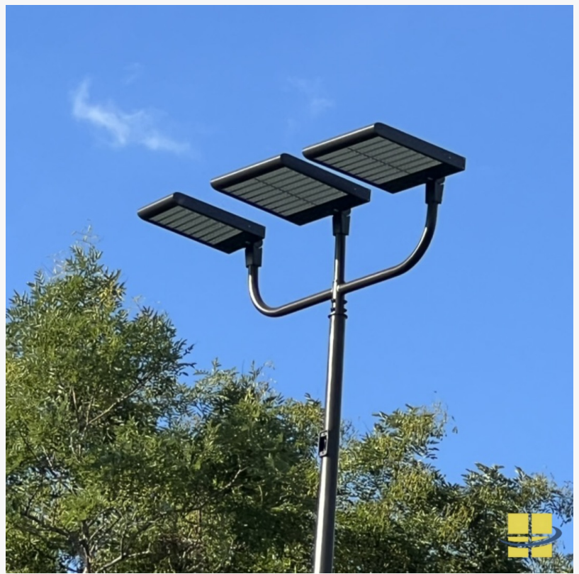
Three Access Fixtures ASTA LED Sports Lights on a triple bullhorn mount at McCarren Park, one of 12 poles lighting the seven-court complex.
