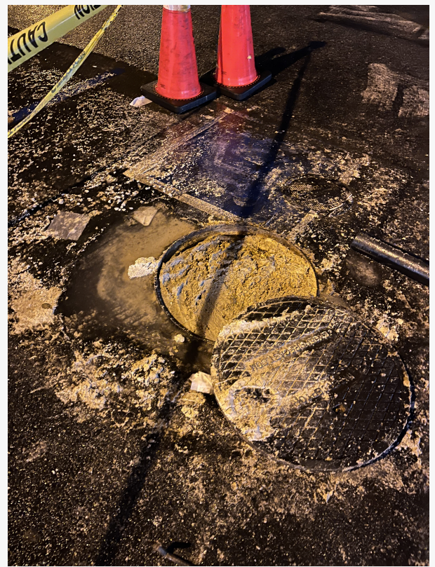
Indoor grease trap overflow showing accumulated FOG requiring prompt professional attention.
