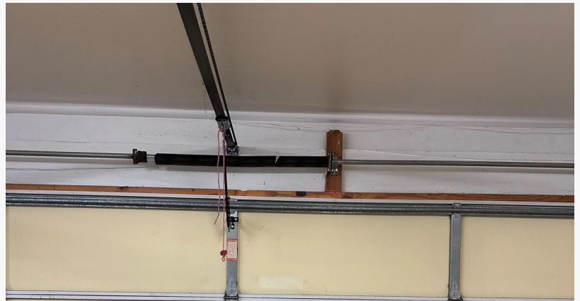
A torsion spring assembly above a residential garage door in Orange County, California.
