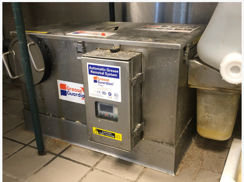
Large professional grease trap installed in a commercial kitchen to capture fats, oils, and grease from wastewater
