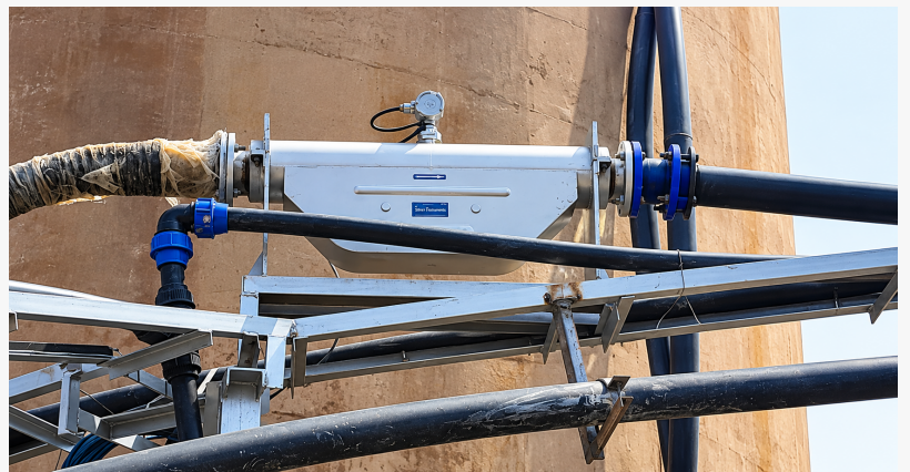
Silver Instruments Coriolis flow meter installed on process piping
