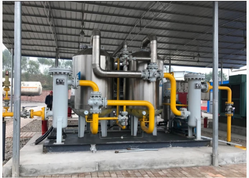
Front Natural Gas Dryer
