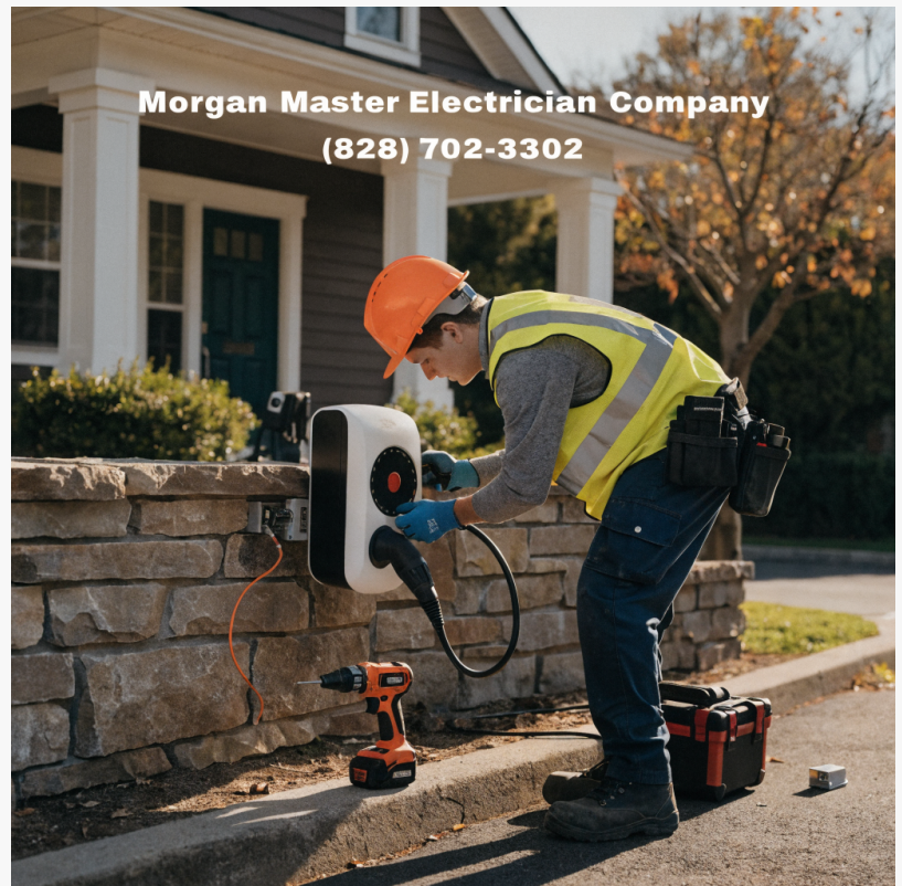
Tesla EV charging station installation in Asheville
