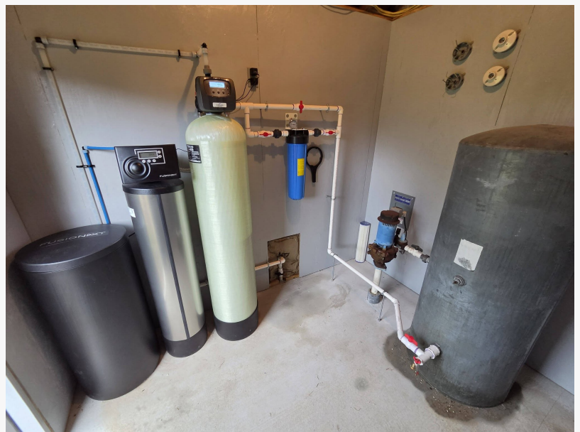
A water softener, filtration tank, and sediment filter installed by Riley Plumbing in Brazoria County, Texas. Softening reduces the minerals that cause scale in water heaters, fixtures, and pipes.
