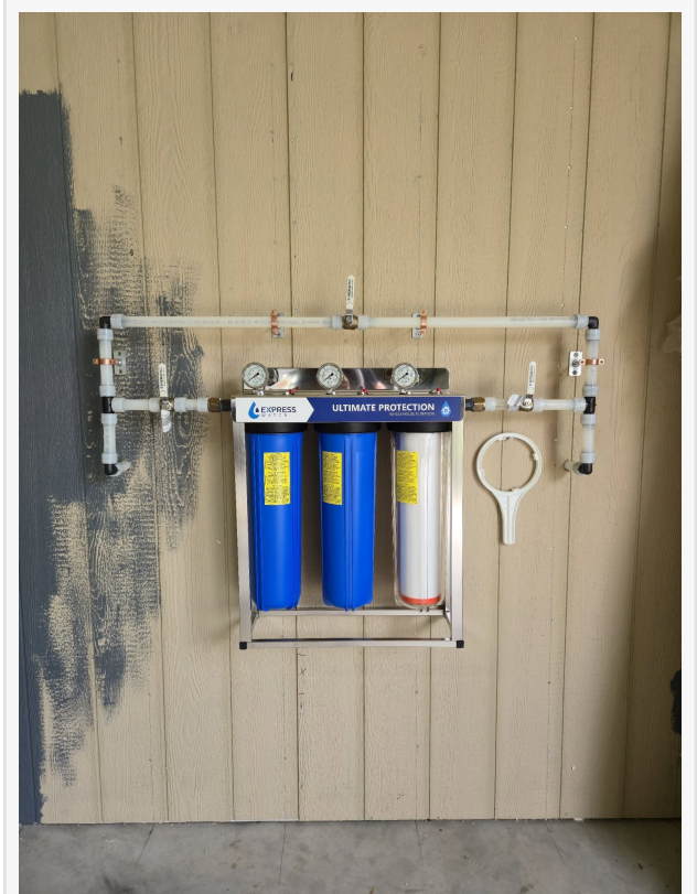
A three-stage whole-home water filtration system with bypass valves and pressure gauges, installed by Riley Plumbing in a new Brazoria County home.
